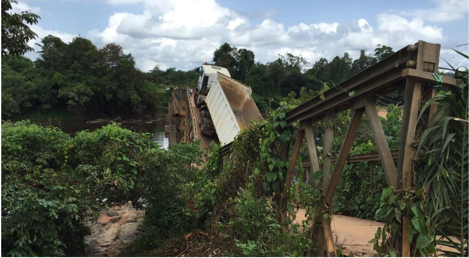
The bridge that connects Rivercess and Sinoe counties, broken from the weight of a truck carrying gravel. Goods can only be transported across the river in small loads via foot or by boat; neither of these options is feasible for transporting planks. This likely decreased the volume of planks coming from multiple counties during the data collection period.
